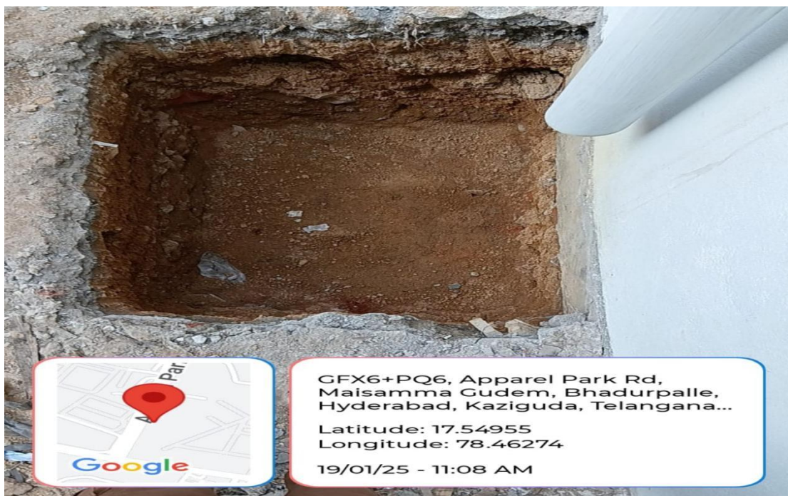
Rainwater Collecting Pits
