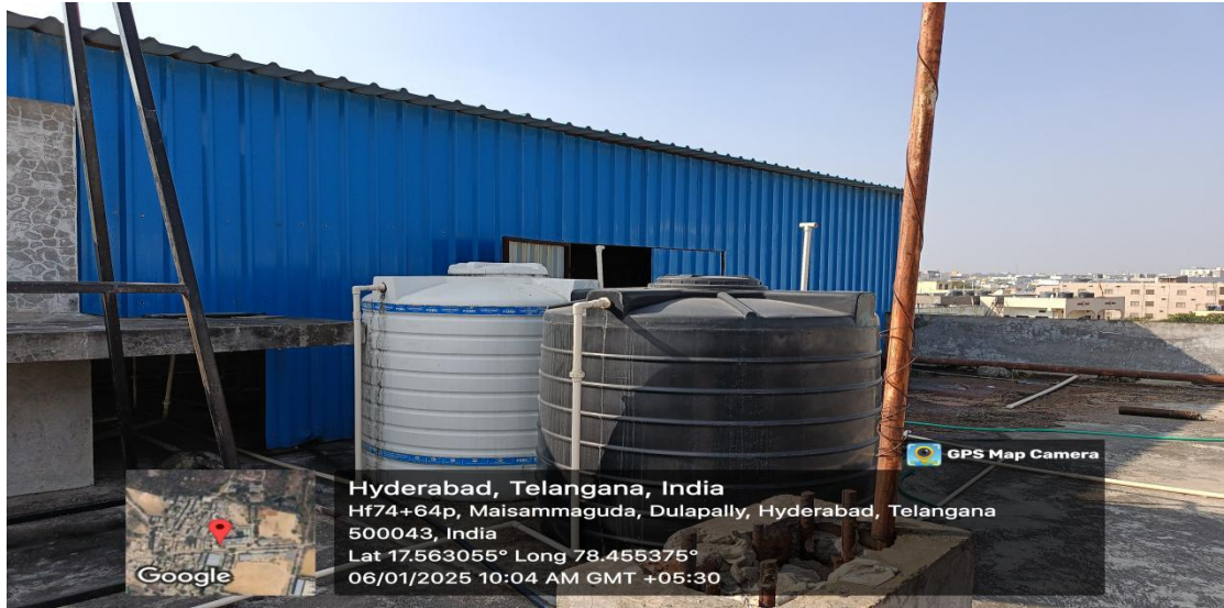
RO Waste Water Collected in Tanks
