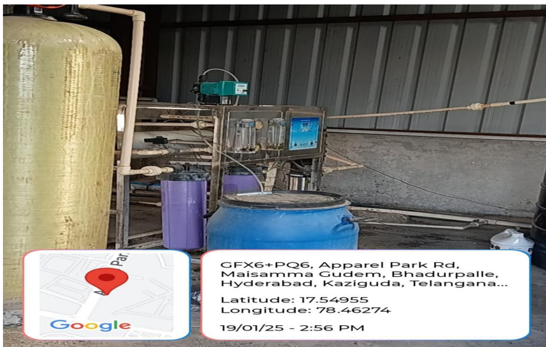
RO Water Plant
