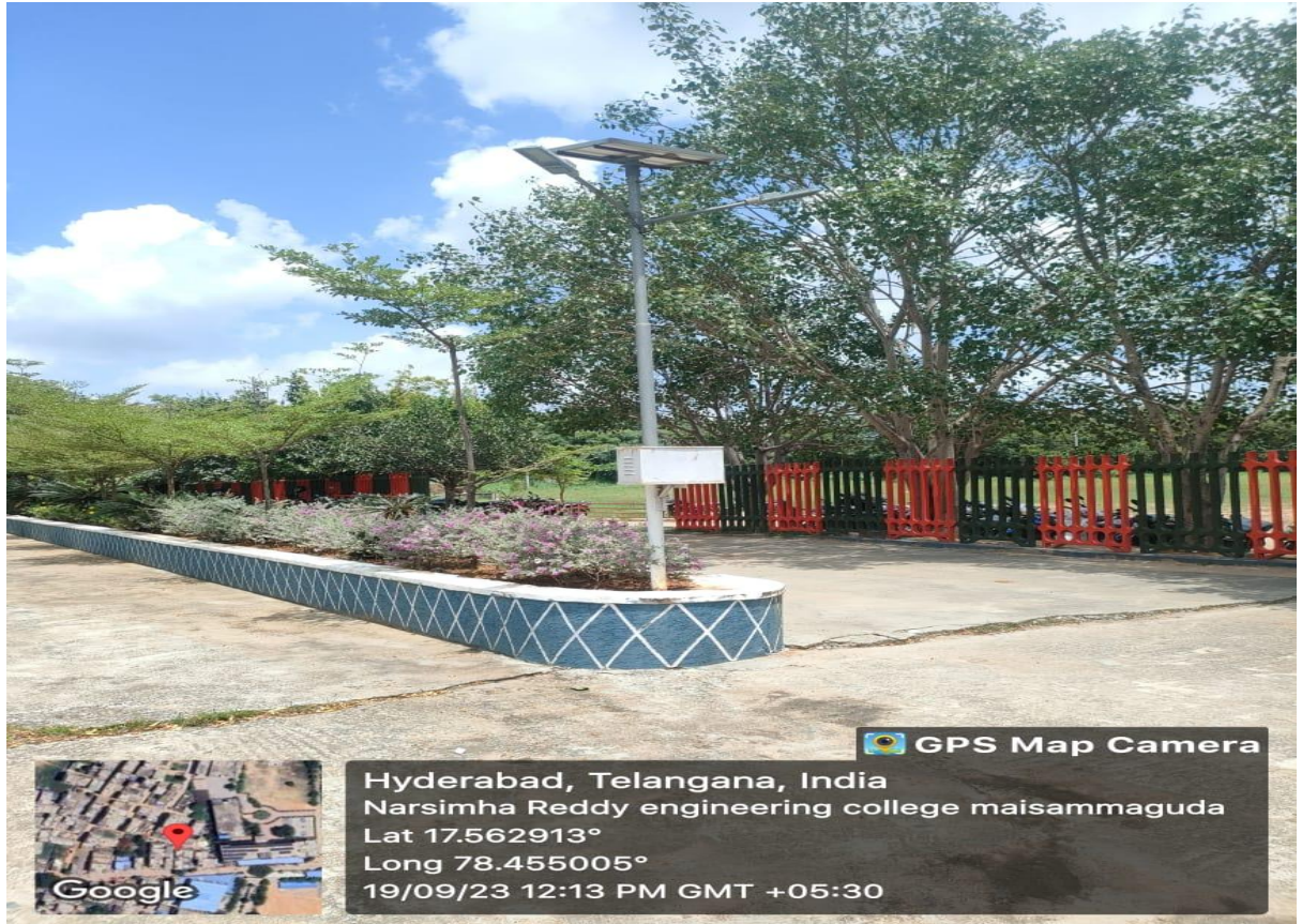
SOLAR STREET LIGHTS INSTALLED IN THE OPEN SPACE OF THE CAMPUS
